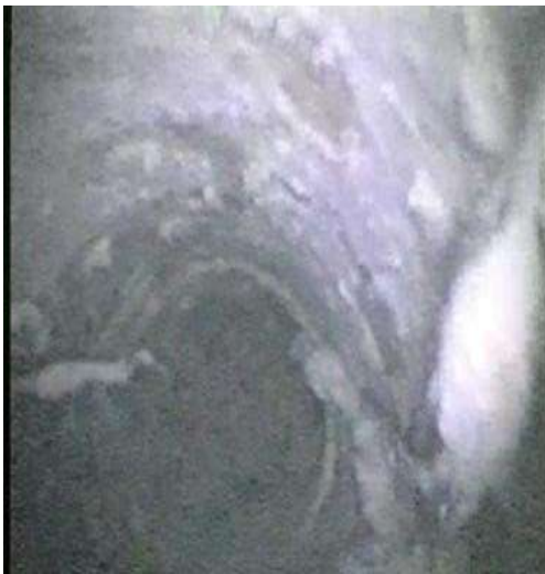
Feed water pipe with sodium hypochlorite
